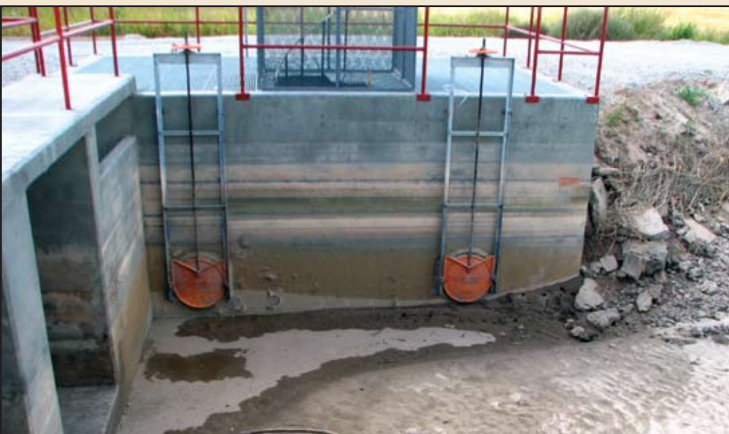
Bypass turbine inflow gates.
