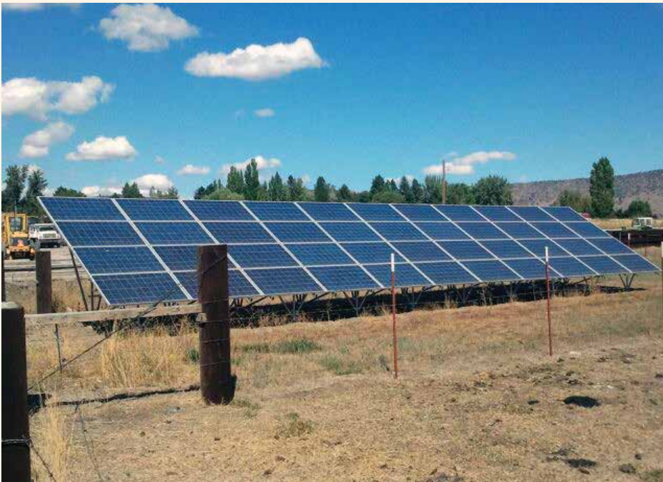
Solar facility at KID's office.
