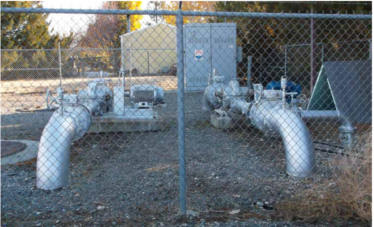
Booster station in Okanogan Irrigation District.
