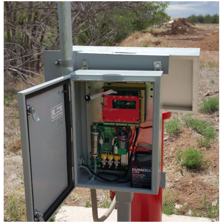
Close-up view of a remote telemetry unit.
