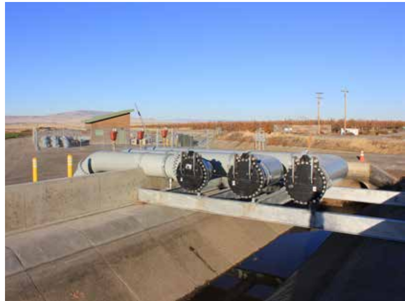
South Columbia Basin Irrigation District's Esquatzel pumping plant, complete.
