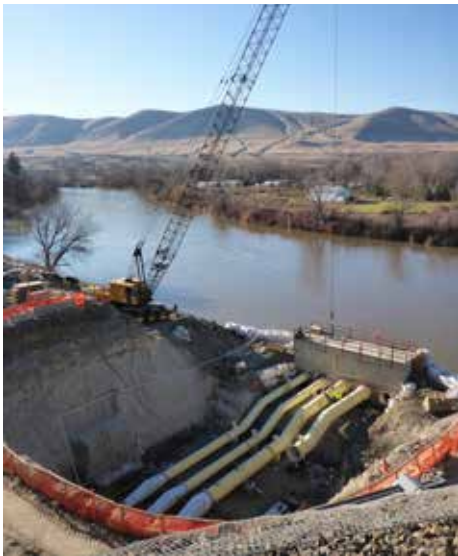
Construction on the Kiona pump station and intake at KID's Red Mountain Local Improvement District.
