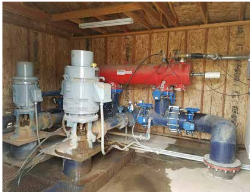
One of NMID's approximately 150 pressure urban irrigation pump stations.
