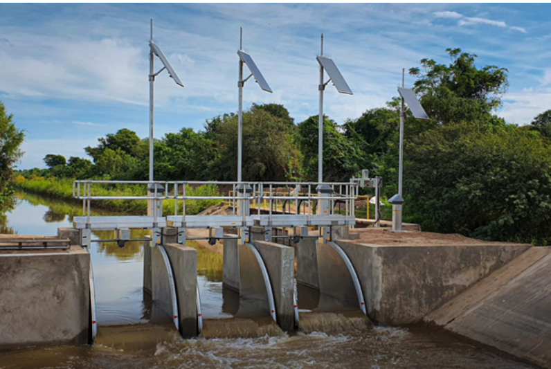
Rubicon gates installed at one of Ledesma's sugar operations in Argentina.
