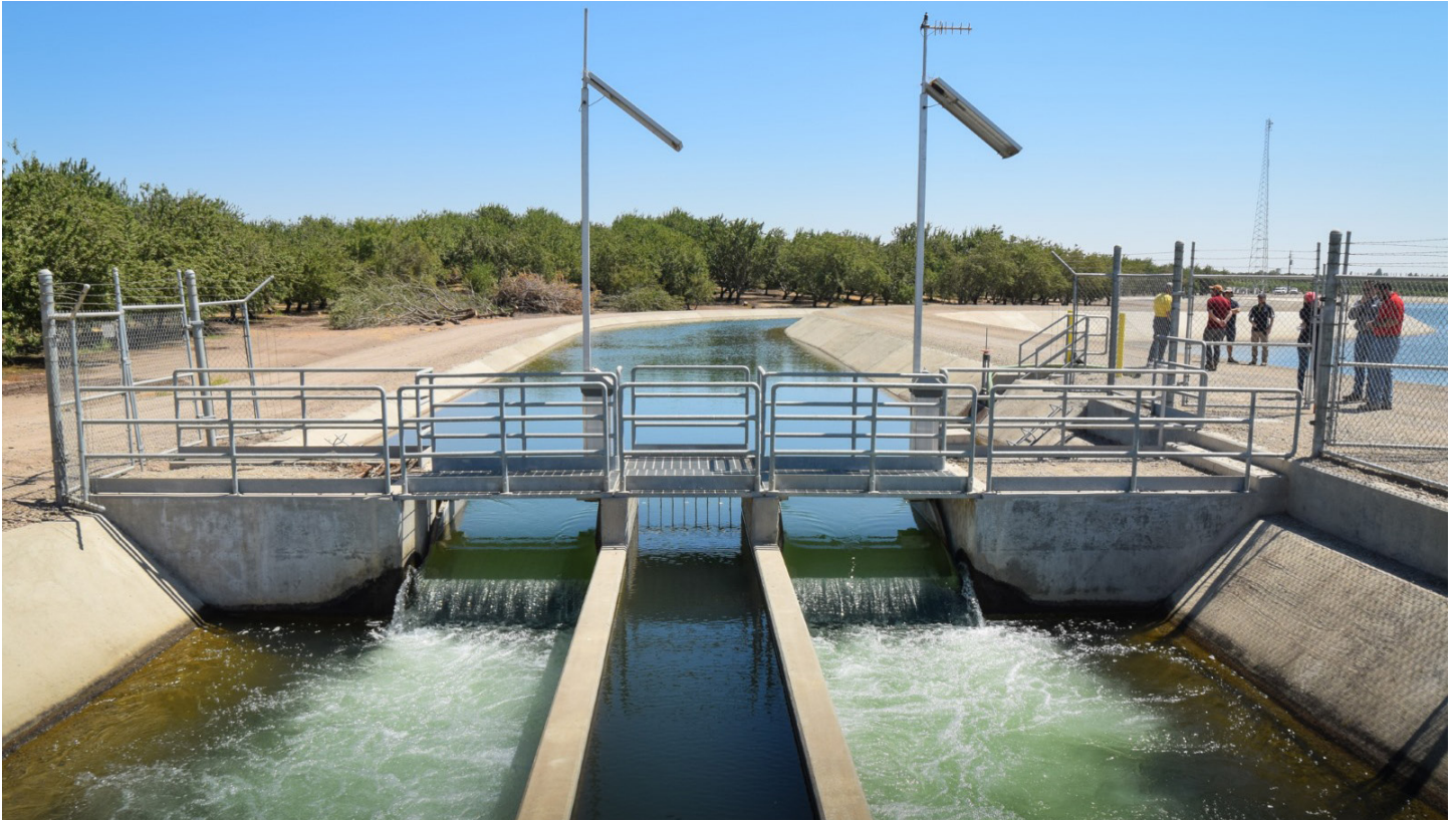
A Rubicon Flumegate installed at an irrigation district in California's Central Valley.
