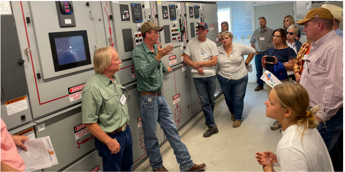
Justin Temple from A&B Irrigation District shows the south-central Idaho group the district's pump station during a discussion of the modernization of irrigation infrastructure.
