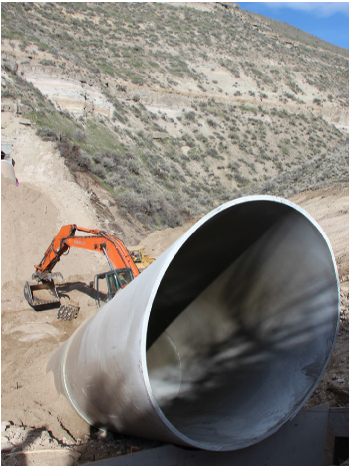
HOBAS supplied a custom-built 96-inch pipe tee along with two custom elbows to create a V-shaped siphon for the Naches-Selah Irrigation District. It also supplied 3,600 feet of 96-inch pipe.
