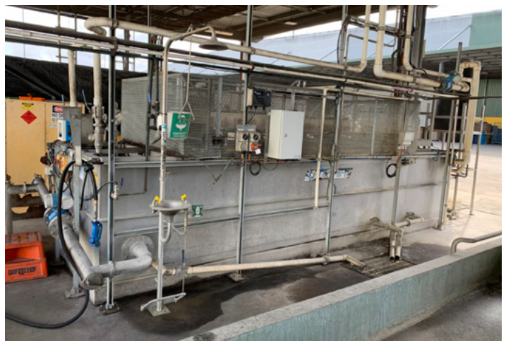
A Streamwise unit installed on a dissolved air flotation system.
