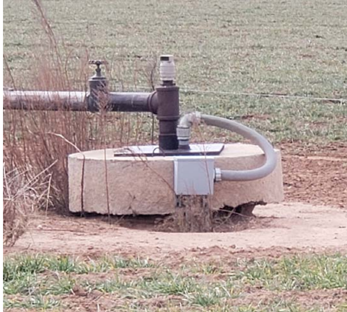
An irrigation well on Danny Fish's farm. The setup includes an above-ground well casing with a discharge pipe connected to a pivot or distribution line; an electrical conduit and control box, indicating a powered pump beneath the casing; and a concrete pad, which seals and stabilizes the wellhead, common for irrigation systems on cropland.
